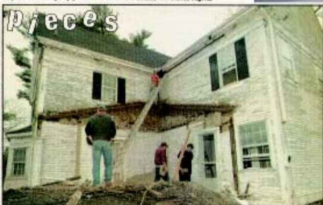
Construction workers with Steve Schurtz Builders continue preparation work Wednesday to save the Becker house in half.
