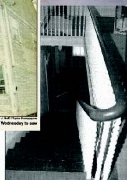
The wooden staircase in the Mansion House leads from the bedrooms to the parlor and living room. The woodwork is reflective of the time period in which the house was built.
