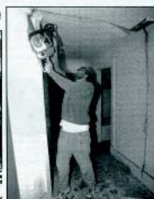
The ripping noise of chain saws sounds through the Mansion House in Fishers Wednesday as Rick Simpson of Steve Schurtz Builders cuts through the upstairs hallway.
